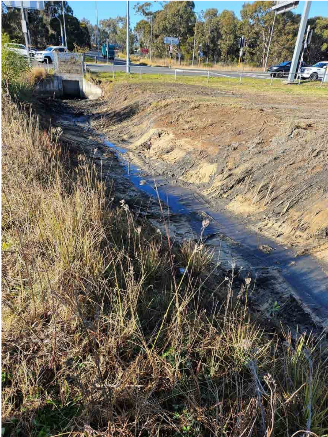
Figure 3.3 Showing excavation works for the drainage channel cut from Rooty Hill Road North south into the BNI, dated between 2020 and 2023. At the time of writing, it is not known which authority authorised these works. The image shows the bank with a cut shallow Blacktown soil profile; a skeletal A1/A2 overlies B horizon clay with evidence of gravels at the horizon interface. (Source: DSMG 2023)
